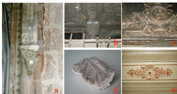
Fig. 1: a: Stuccoes of stage box affected by the fire; b, c: Stuccoes of Foyer covered by a layer of combustion deposits; d: Piece of stucco fallen from the stage box decorations; e: Golden stucco in area not affected by the fire.
